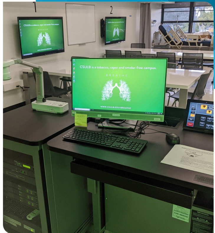
The instructor's podium includes a Extron touch panel to toggle displays and control other AV systems.
